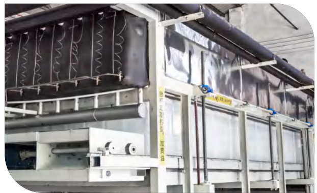
Commissioning site of 30t automatic ice block ice machine
