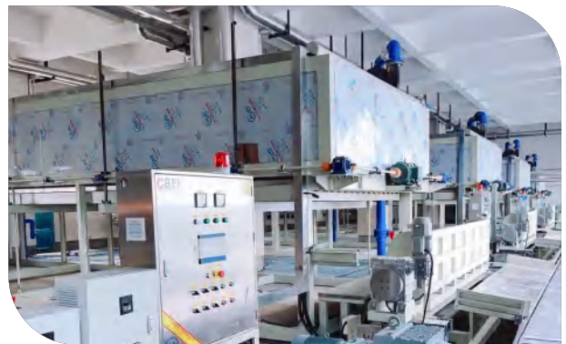
Commissioning site of 160t automatic ice block ice machine
